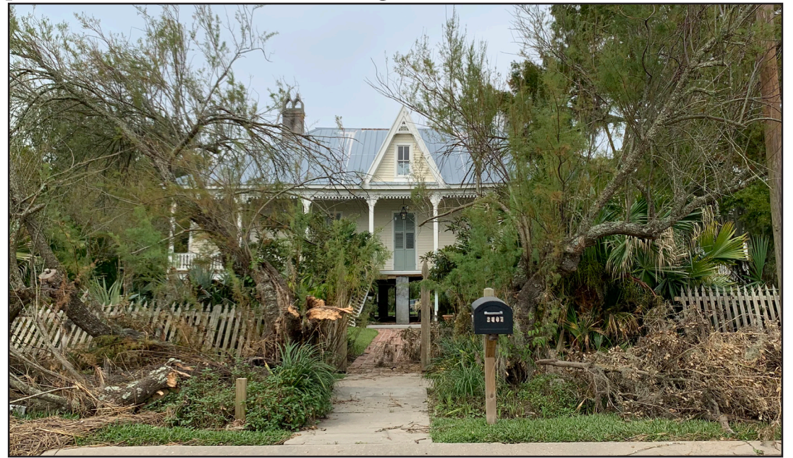
Photo courtesy of Abby Pucik Storm damage of the Pucik house after Hurricane Ida
